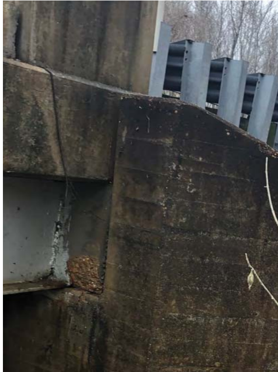
Corrosion and Decay at Girder Connection to East Abutment on Inlet Side
