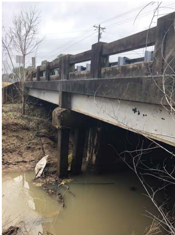
Extensive Decay of Pier near Girder and Foundation at Inlet
