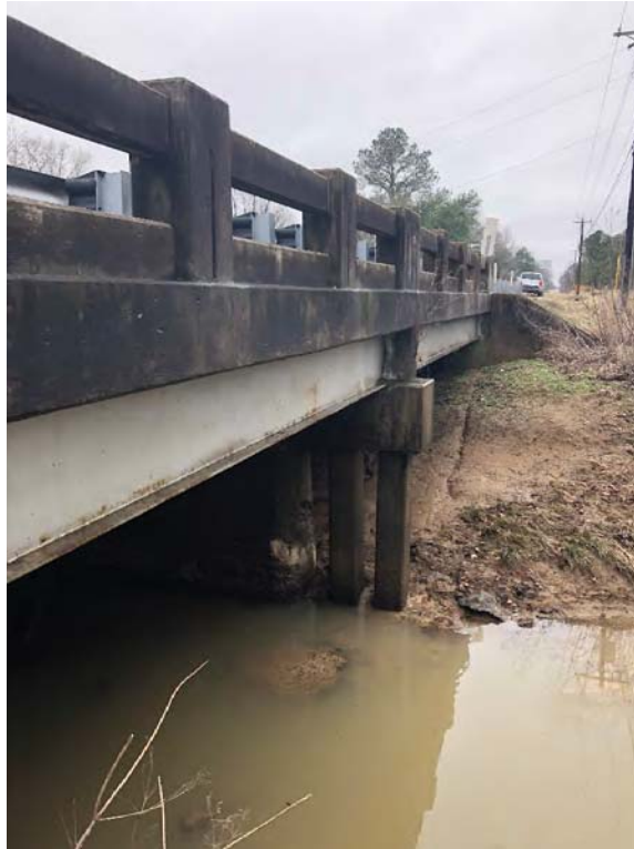
Corrosion on Girder at Outlet
