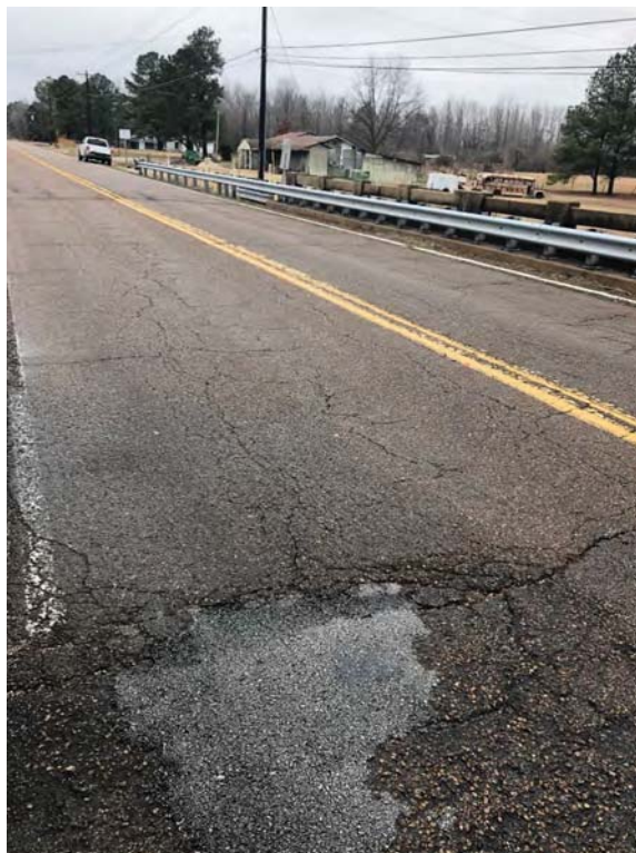
Extensive Pavement Cracking and Rutting on Bridge
