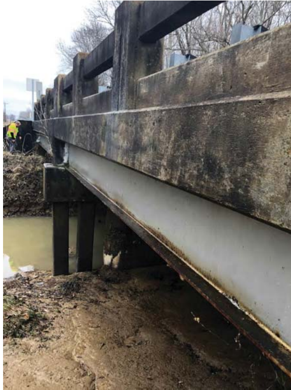
Corrosion of Outlet Girder between West Abutment and Pier
